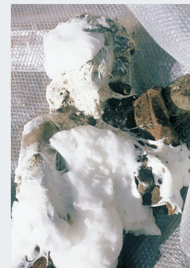
Sl.3. Zatečeno stanje Anđela - detalj, fotografija prikazuje infestaciju skulpture bijelom plijesni i gljivicama (dokumentacija HRZ-a) Pic.3. Prior condition of the Angel - detail; the photograph shows infestation of the sculpture using white mould and fungi (documentation of the Croatian Conservation Institute)
